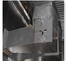
New OFA Nozzles on Boilers "A"
