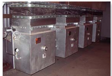
OFA Nozzles on Boiler "C"
