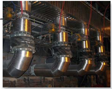
New RDF Fuel Distributors with Air Supply on Boilers "A"
