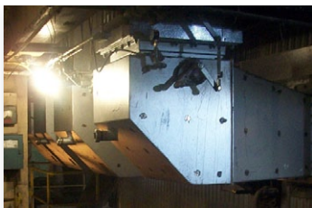
OFA Nozzles on Boiler "B"
